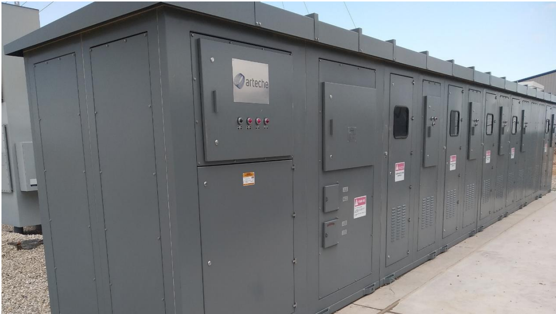
Metal Enclosed Multistep Harmonic Filter in Sendero Midstream – New México
