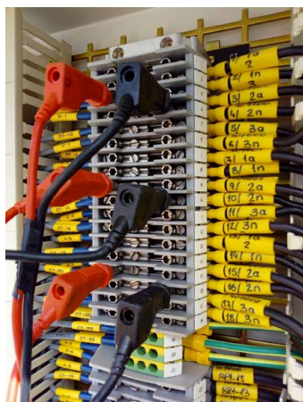
› Access to the Marshall box
